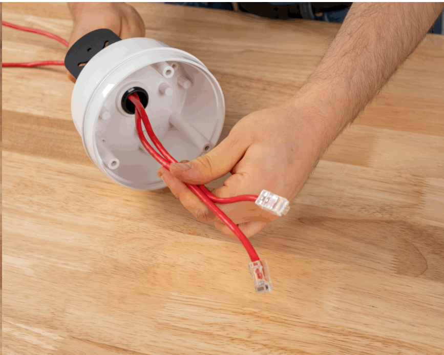
View of cable for service loop
